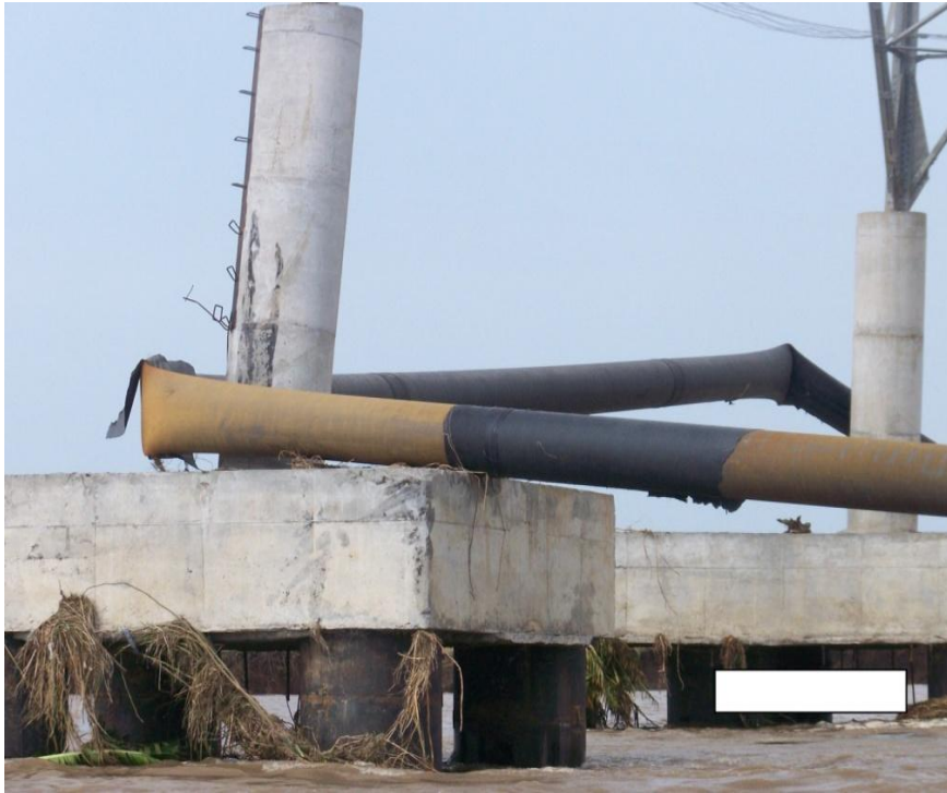
Torrent Transmission tower on the south bank of the Narmada River
