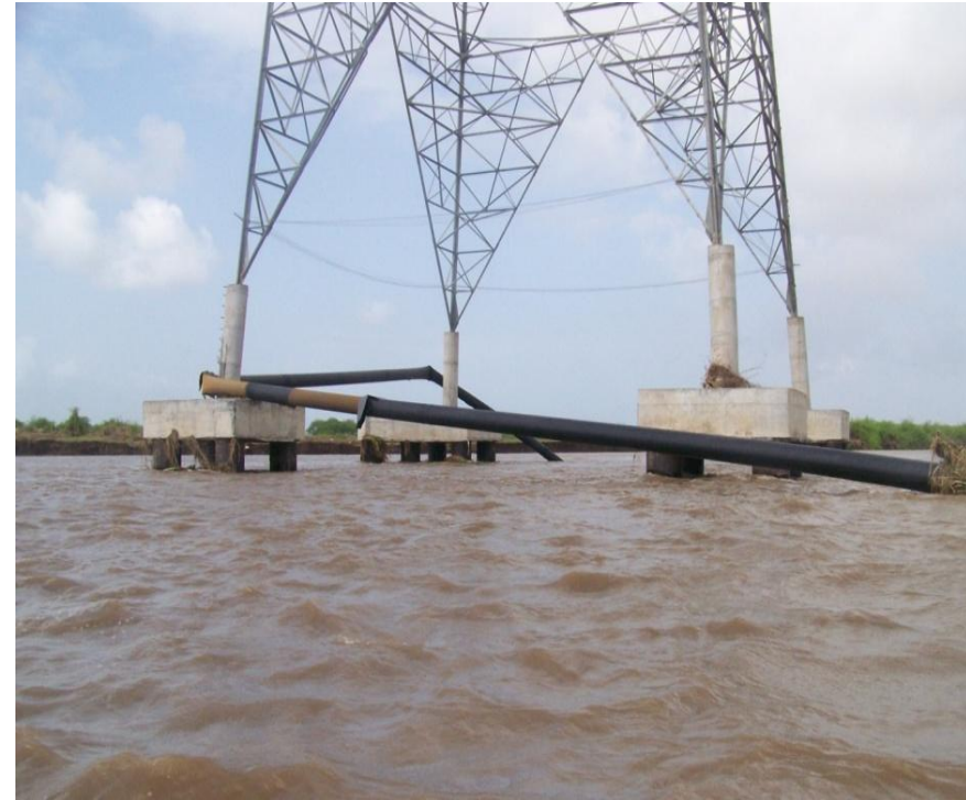
Transmission tower on the south bank of the Narmada River: It was on land but now it is in 10 m depth of water due to erosion.
